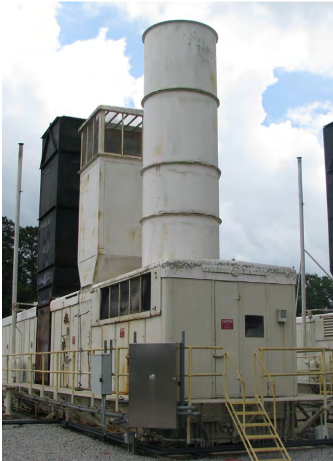
Parr Combustion Turbine
