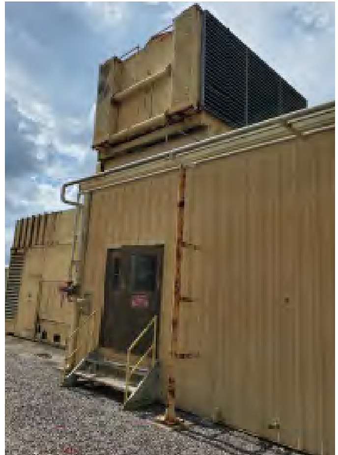
Bushy Park Combustion Turbine
